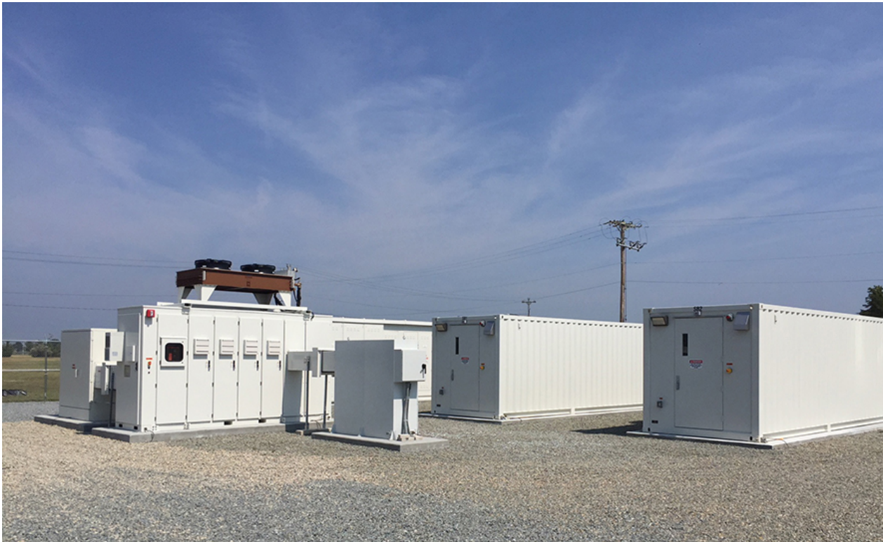
Featured is the Battery Energy Storage System yard for the Microgrid that supports the critical power functions of the Otis Air National Guard Base. East Penn and Ecoult are proud to have a role in this important use of its battery and battery system technology.
